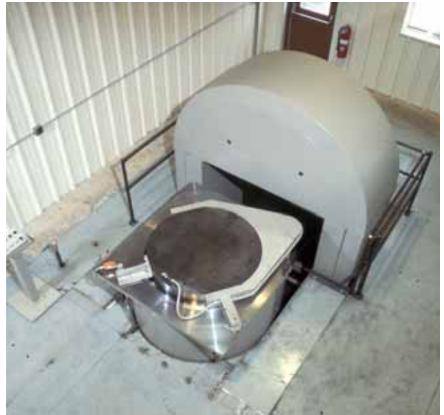
Quintus Model QIC 44-78.7-36 Installed at a midwestern manufacturing plant. Vessel dimensions: 44" dia. x 78.7" high. Operating pressure: 36,000 psi.
