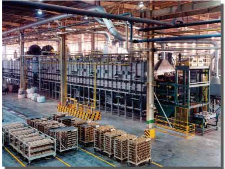
3a. Fully automated Sand Lion roller hearth system T-6 heat treats and age hardens over 4,000 kg/hour of aluminum engine blocks. The system replaced an older multi-step process and paid for itself in 18 months with demonstrated energy savings, reduced floor space, environmental controls and sand reclamation.
