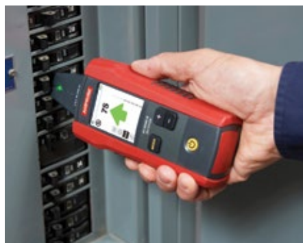
Identify the single correct breaker
