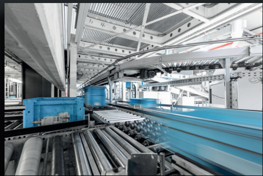
Indoor materials handling
