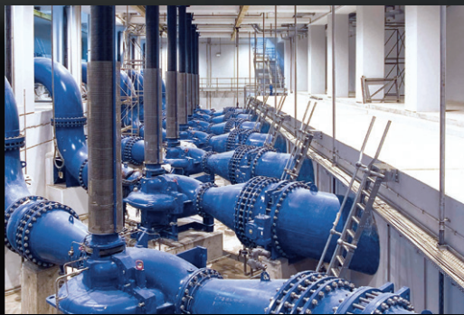
Pumps and compressors
