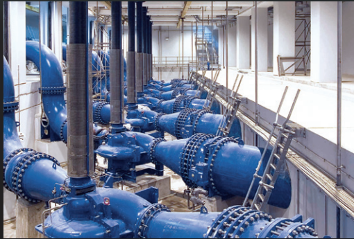
Pumps and compressors
