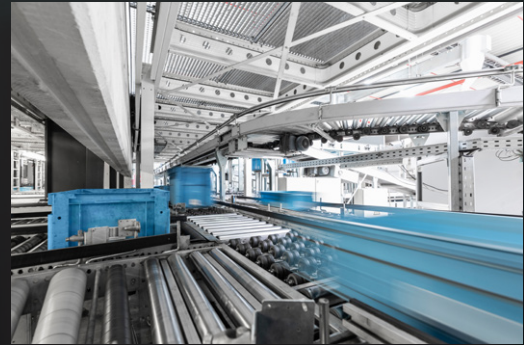
Indoor materials handling
