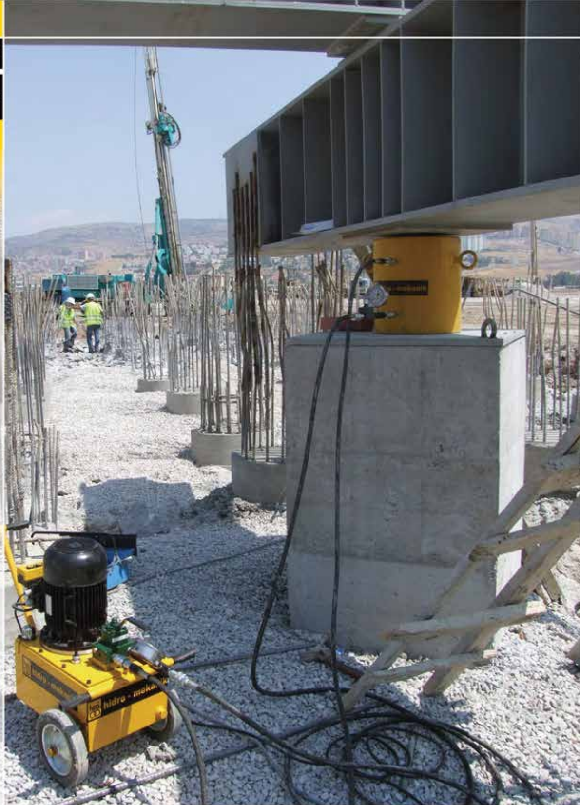
PILE TEST HYDRAULIC SYSTEM
