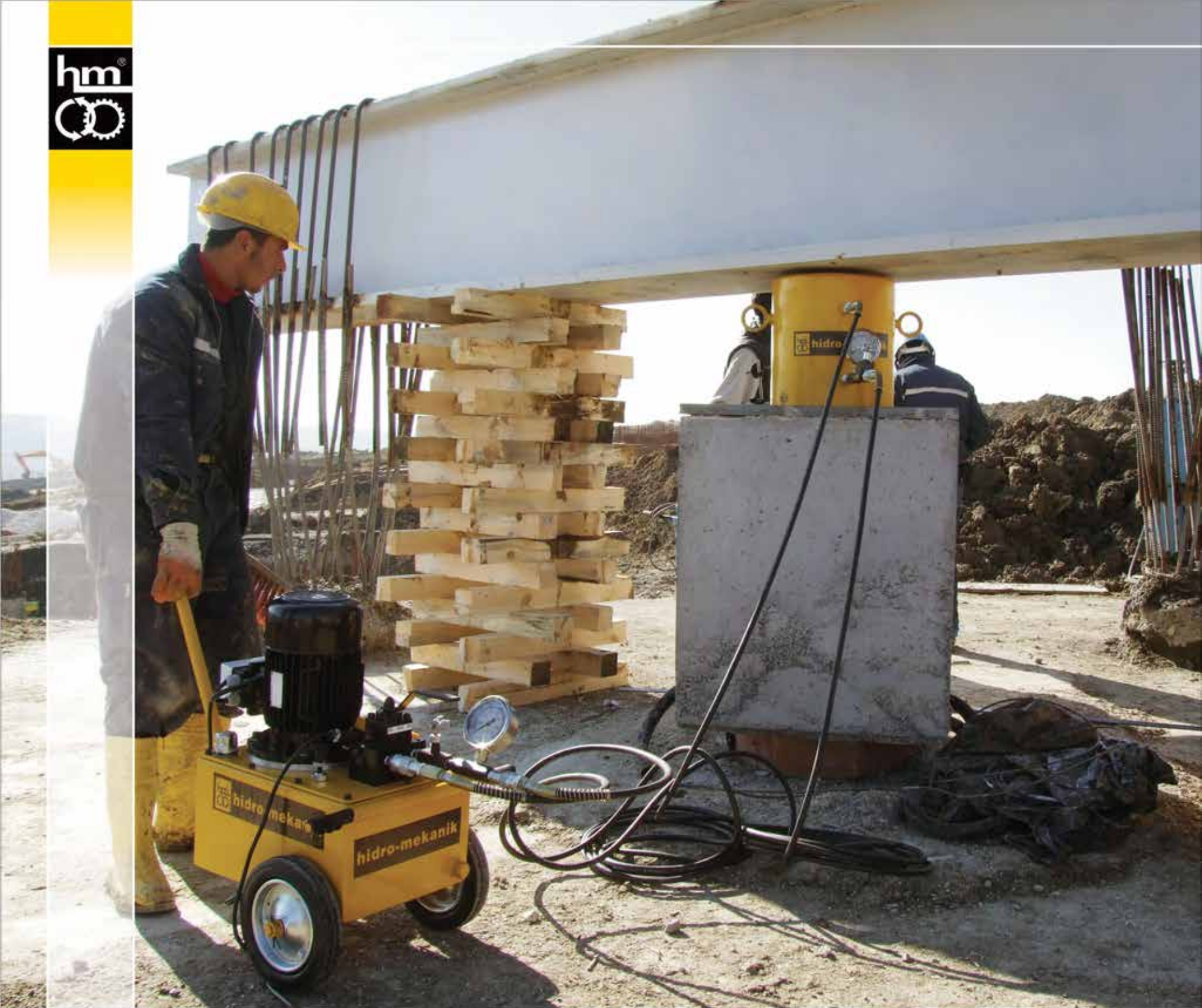
PILE TEST HYDRAULIC SYSTEM
