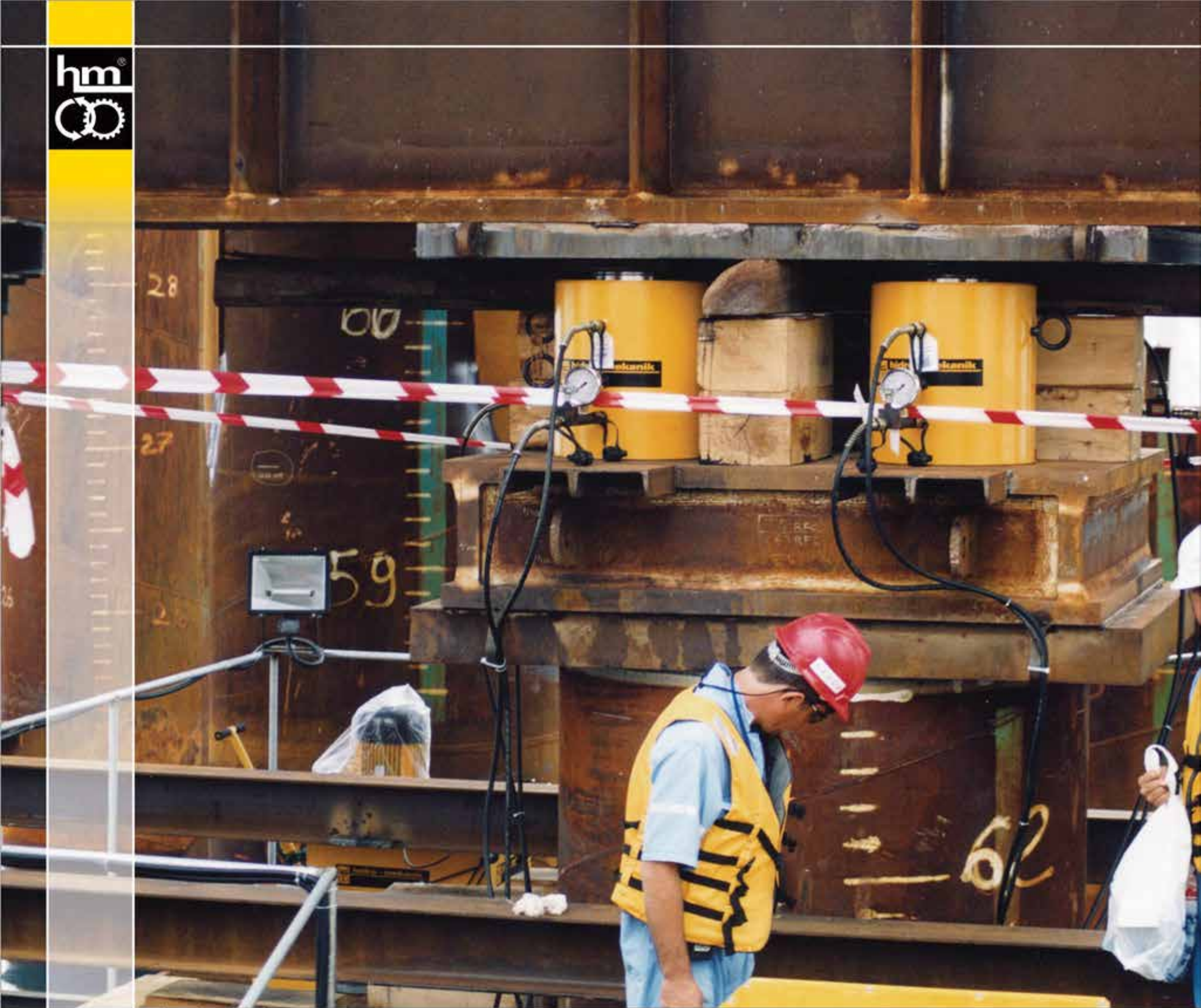
PILE TEST HYDRAULIC SYSTEM
