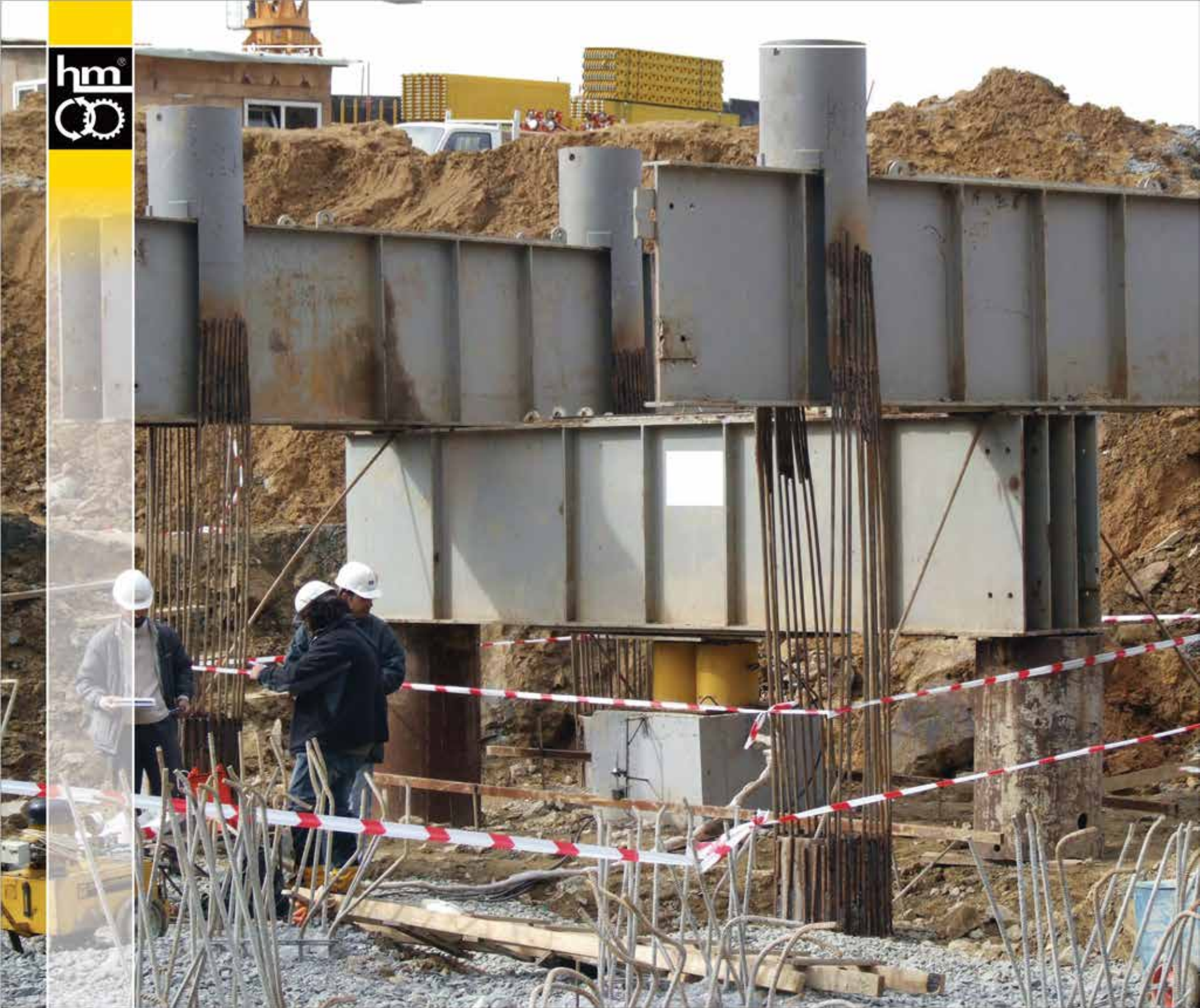
PILE TEST HYDRAULIC SYSTEM
