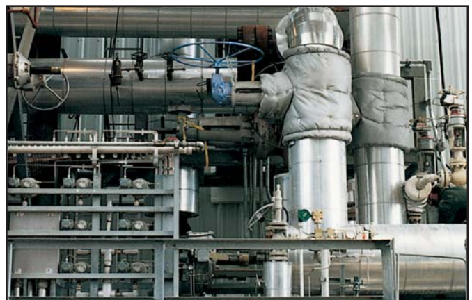
Pressure seal valve in a cogeneration power plant.
