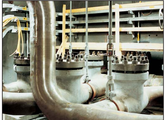
Pressure seal check valves installed in a nuclear power facility.
