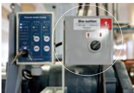
Die setter operation panel
