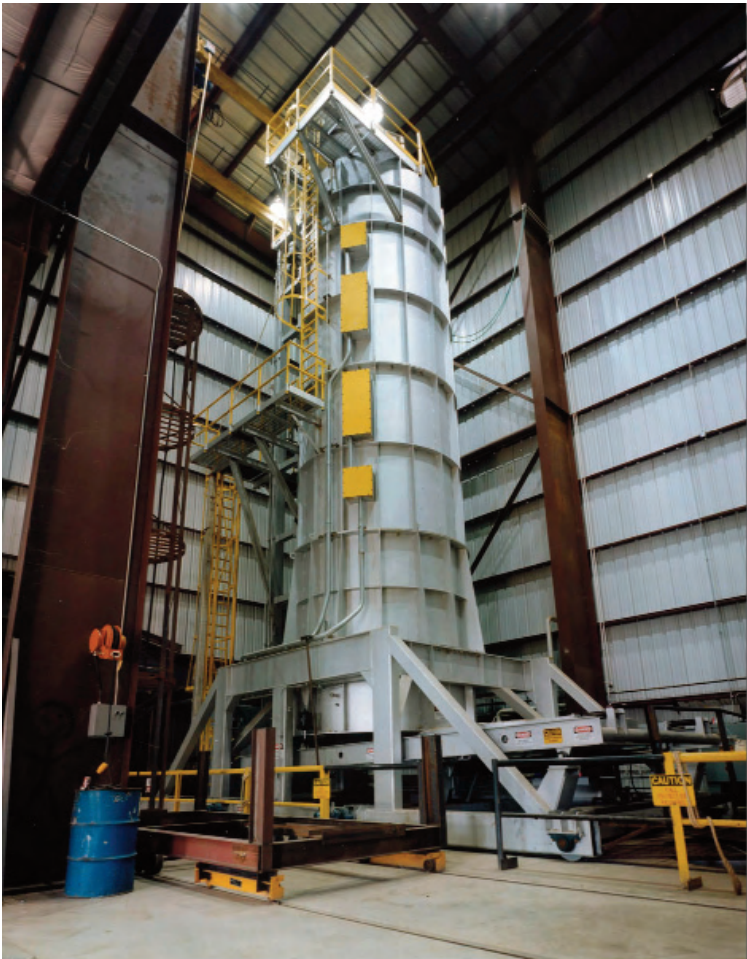
4b. Mobile quick quench tower furnace for solution heat treatment of 32' extrusions is complete with an in-floor glycol quench system and load area.
