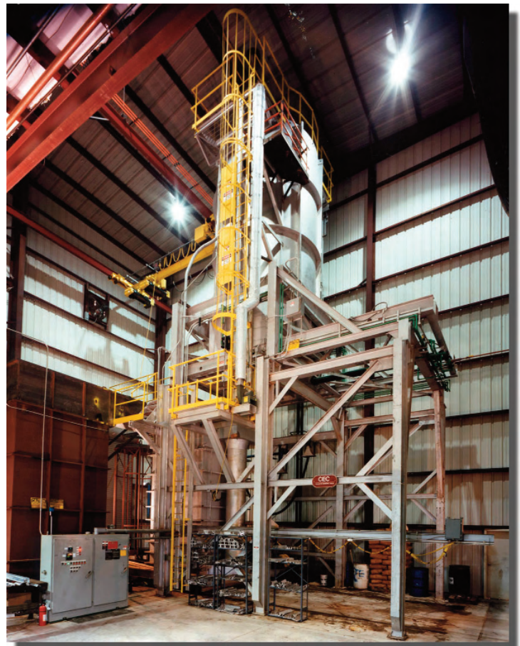
4c. This drop-bottom furnace processing 16' extrusions is complete with a mobile transfer car and poly (alkylene) glycol quench system.
