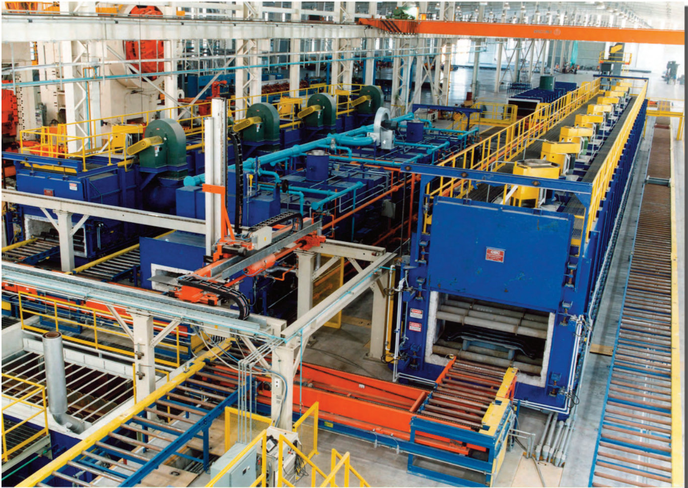
6b. Complete heat treat facility with harden, quench and temper, normalize and slow cool capabilities for production of 25,000 lb. per hour of crankshaft and suspension forgings.
