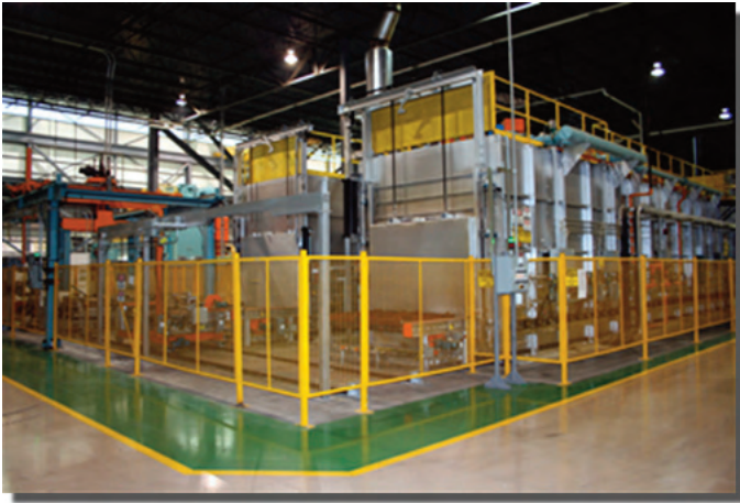
8a. Continuous T-6 heat treatment of forged aluminum automotive components with gantry stacker and with process data acquisition and retrieval.
