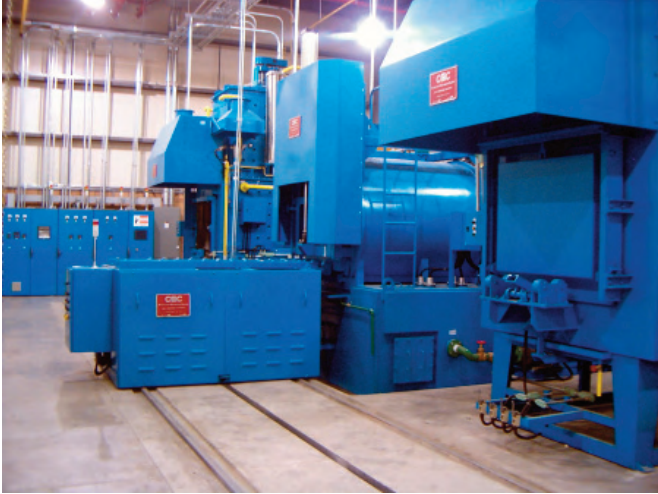
3a. Complete Flexcase model 364832 line with IQ Furnace, Vacuum washer, Tempering Furnace, Charge car and supervisory control system
